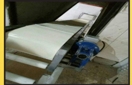
Cold Storage Conveyor
