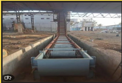
Bagasse Handling Chain Conveyor
