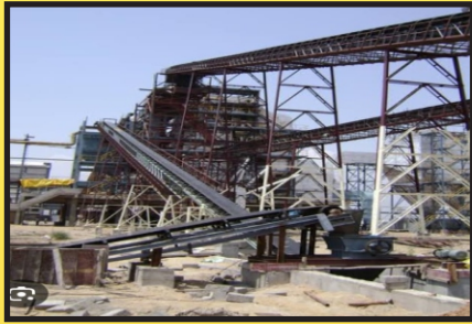
Boiler Fuel Handling
